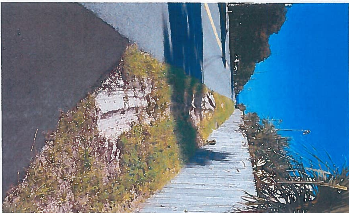
Picture 3: West side of Nautilus Road Right of Way in front of Hidden Lagoon racetrack.
