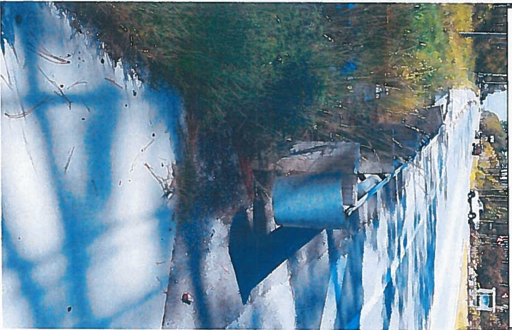
Picture 5: East side of Alf Coleman Road looking south. Guardrail near Harrison Walk Subdivision where storm pipes are to be extended and new headwall constructed.
